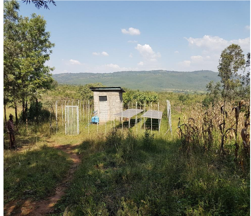
Drip irrigation system powered by solar energy installed in Ampo Koysha, Wolayta, Southern Ethiopia
